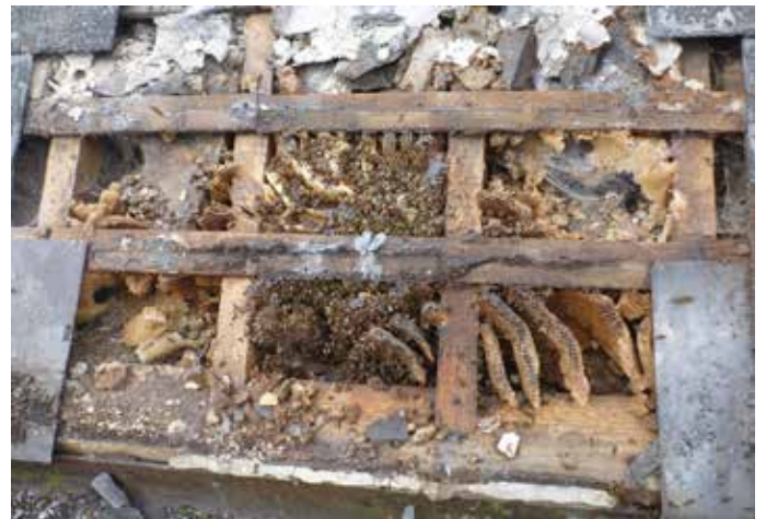
Figure 7: An example of a bee colony in a roof beneath thin stone slates.
